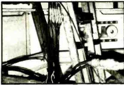
Figure 6. Microphone cables were gathered underneath the tree's wooden flooring and carried to the splitter box area at the monitor mix position on multipair runs.
