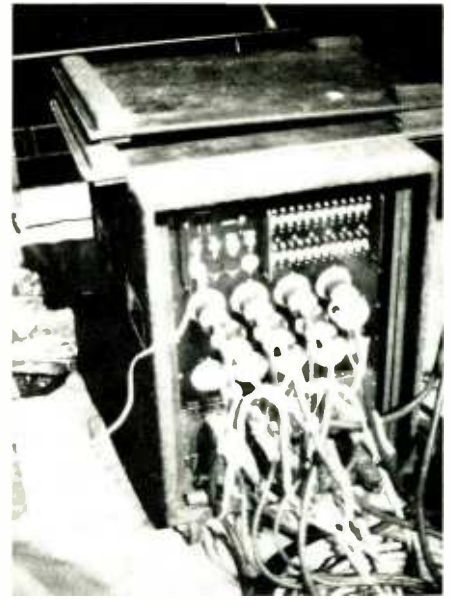
Figure 14: A regulated power distribution system offers each mix and stage equipment area two 20-amp legs of AC power.
