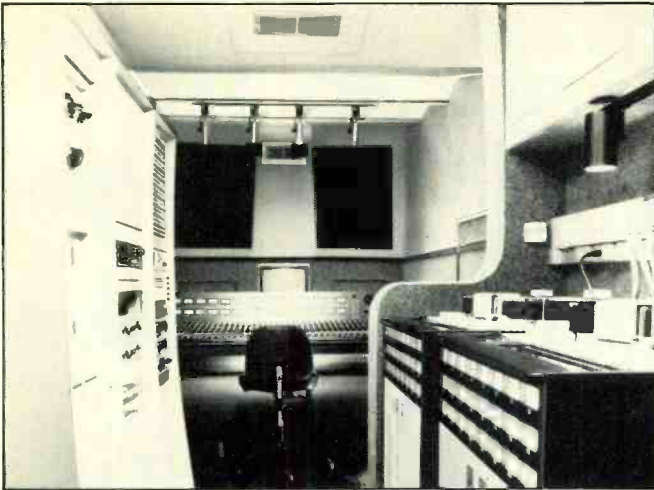
WESTWOOD ONE: two Ampex MM1200 24-track and ATR102 2-track tape machines; MCI JH-636 Series console with 36 inputs, and Sphere 1604 sub-mixing system; monitor system is two Altec 604Es in custom DeMedio cabinets with Mastering Lab crossovers. 9540 Washington Blvd., Culver City, CA 90230. (213) 204-5000.
