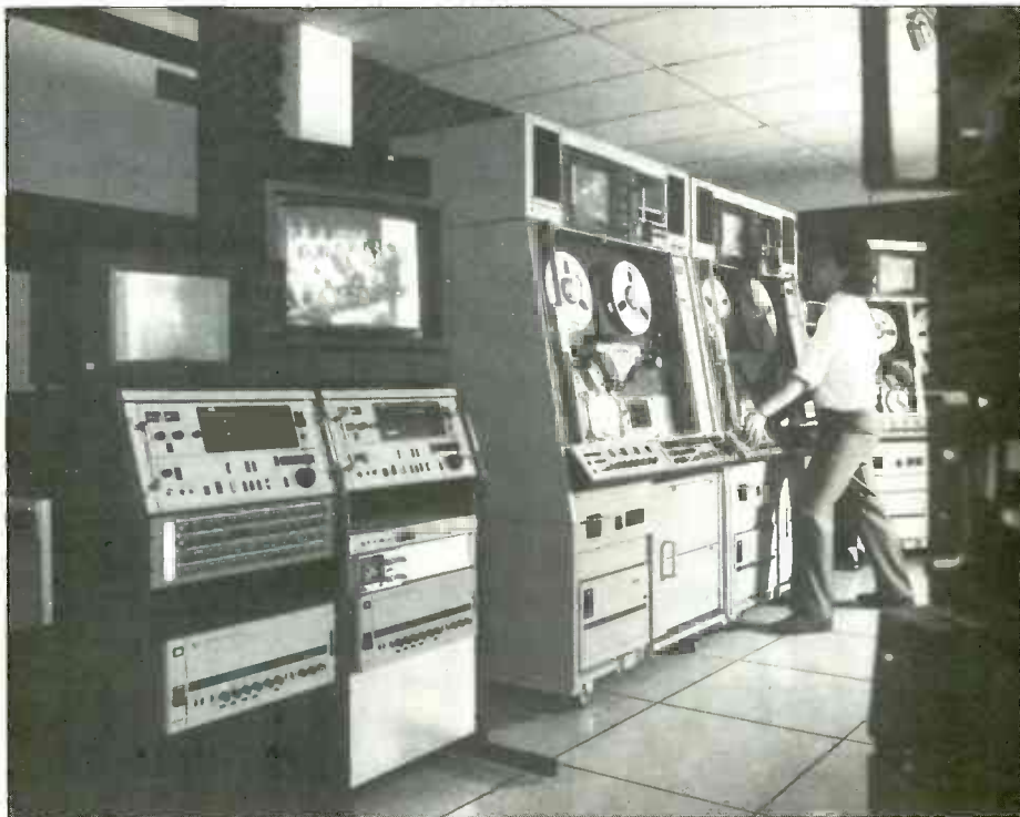
Central control room
