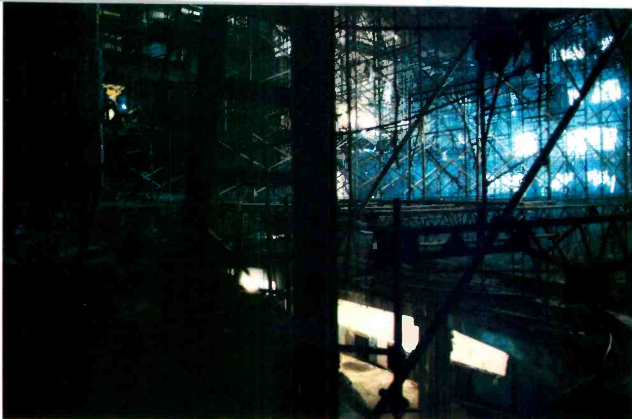
The interior of Avery Fisher Hall looked almost bombed out during the recent reconstruction. The New York Times reported that all the suitable scaffolding on the East Coast had been rounded up for the job. Below, a worker passes through what was once a door in the auditorium's reinforced concrete rear wall, the thickness of which made the eventual task of tearing it out a difficult one.
