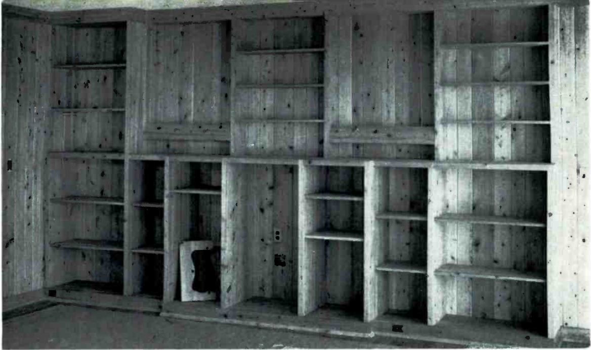
Fig. 3. The entire installation was planned when the architect's drawings were made. Built-in bookshelves and cabinets were to line one wall of the living room, as shown above. Provision was made at that time for the installation of a complete music system for the entire house.
