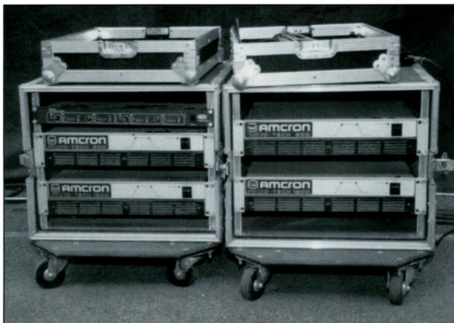
Figure 6. These are the power amps for the local system at Niamey Stadium. (Amcron is the outside the U.S. name for Crown.)
