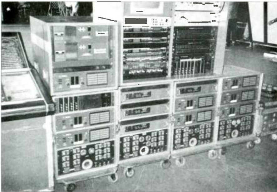
Figure 4. Power amps, equalizers, limiters, etc., used for the Alabama show.
