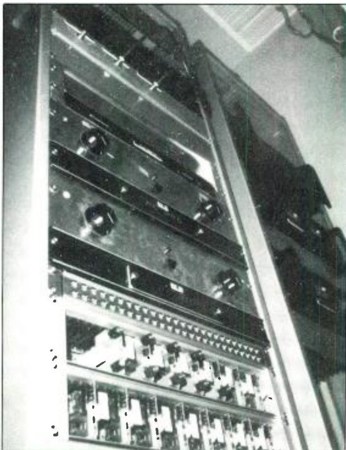
High-level room rack, featuring Crown, UREI and Yamaha power amps.
