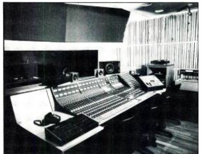
Control Room B featuring a Neve 8068 console, Studer A-80 VU MK III & 24-track tape machine, UREI Time-Aligned™ monitors, and LinnDrum.
