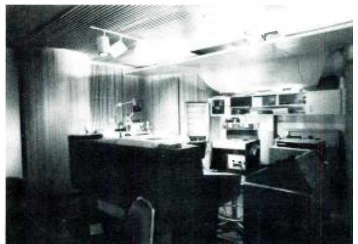
Rear view of new mastering room showing side wall polycylindrical absorber/diffusers, ceiling cloud, and rear wall cabinetry enclosing mastering computer. Grillwork on ceiling and walls is also shown.
