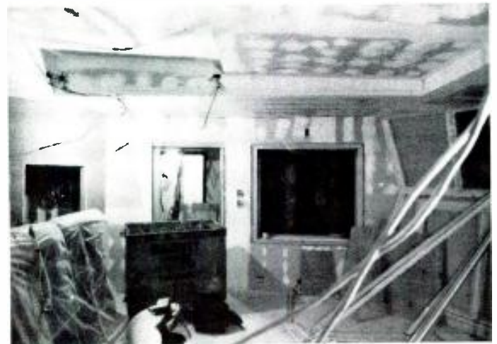
New mix room under construction. On the left is the polycylindrical auxiliary equipment enclosure and the MCI 56 console (wrapped in blankets). On the right is the left monitor enclosure and the vocal room window (through which the MCI console was delivered).
