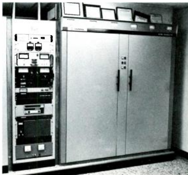
Signal processing and control electronics, with the 10 kW transmitter on the right.
