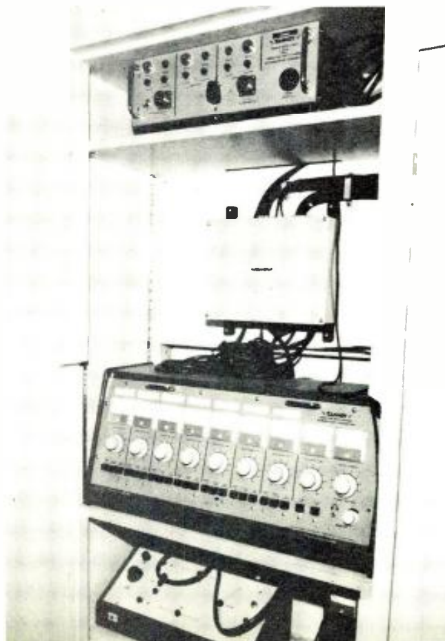
Figure 2. The equipment used to drive the auditorium sound-reinforcement system, and for the r.f. amplifier loop used for simultaneous language translation in the auditorium.
