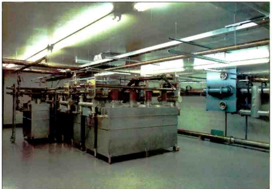
The combiner room of the tower in 1985, when only five FM stations and one TV station were broadcasting from there. The "pipes" are large-diameter coaxial cables.
