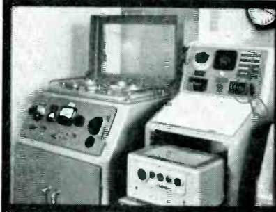
Quality Check Room. Programmes originating from abroad are here passed through a QUAD control unit and power amplifier where they are filtered and balanced for optimum quality prior to transmission.
