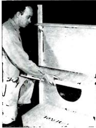
Fig. 4. Installing the center shelf. Note that two pieces of 1 \times 1 have been attached to the shelf before mounting on the front panel.
