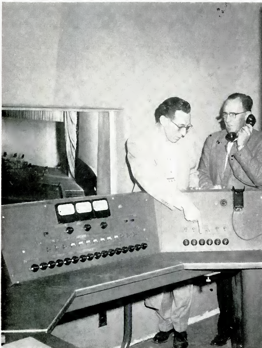
Fig. 7. Tom Roseberry, of Roseberry & Son, points out some of the features of the control console. Telephone communication is provided throughout the building from the control room, linking all production and operating facilities.
