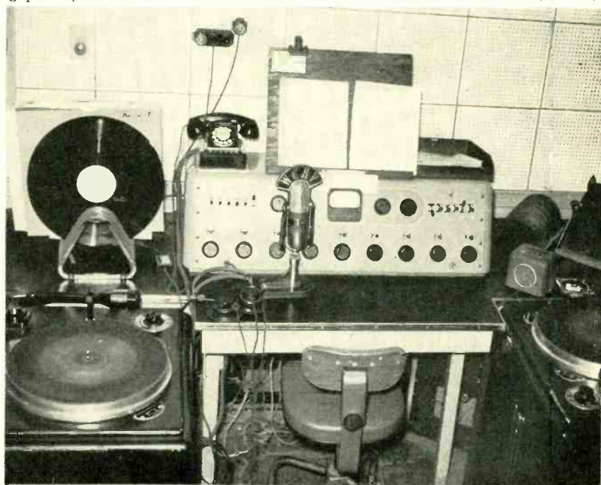
Fig. 1. A control room operated by announcers. Notice the wooden copy rack which has been added to the console, the records to be played, and the telephone which the announcer answers after business hours. In such installations microphone placement is always a problem.
