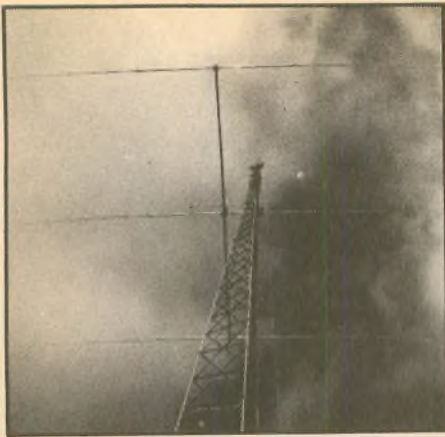
From atop the tower Earl gives the 80M beam a helping hand on its way up the tower
