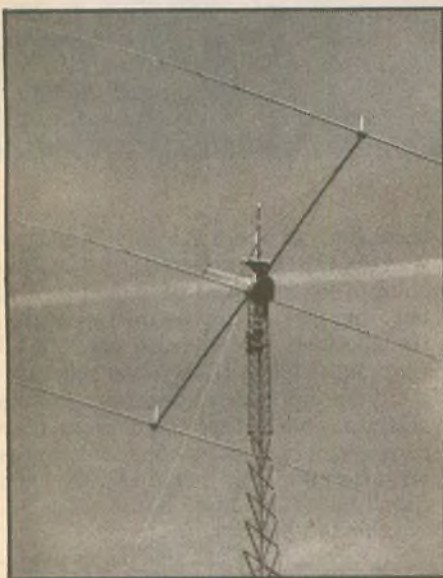
Way up there! Earl stands on top of the tower platform while Gary stands just below, preparing to bolt the 80M beam to the mast
