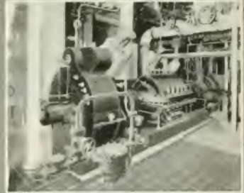
Turbine and Centrifugal Boiler Feed Pumps
