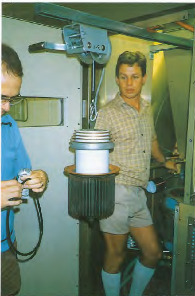
Lifting facility Continental Electronics transmitter for tube change. Barrie Morton (R) Mgr NT supervising operations.
