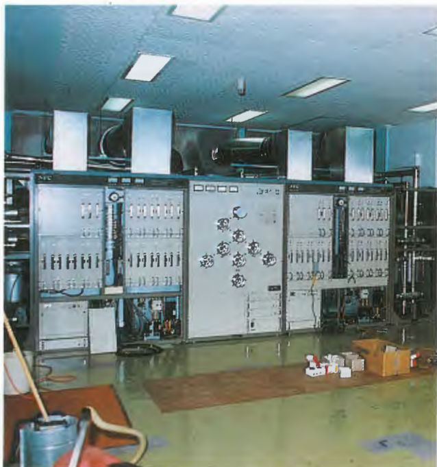
UHF National transmitter at installation stage.
