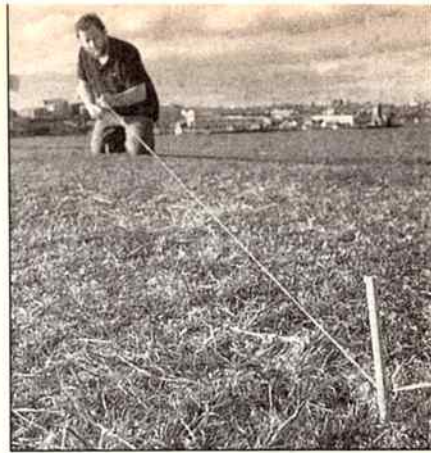
With the surface for the quad element pegged-out on the ground, run string diagonally between opposite corners, marking the centre where they cross.
