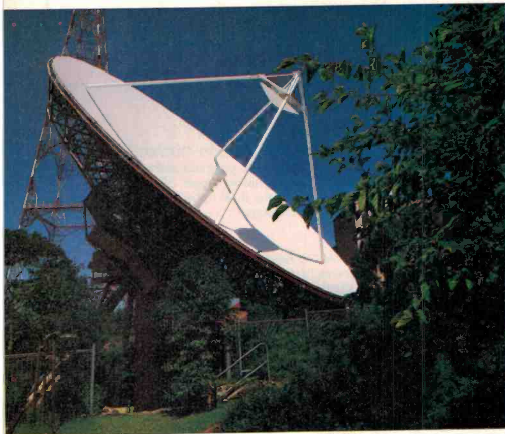
A large commercial installation like this will send TV signals up to Aussat. It can also receive signals sent to the studios via the satellite.
