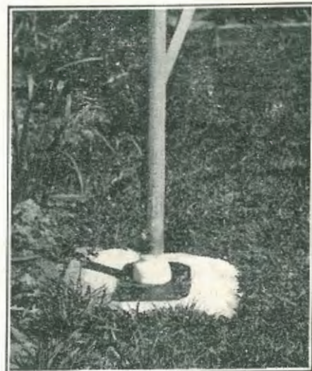
Fig. 3.—The base of the mast rests on a white porcelain (petticoat type) insulator, which is let into a block of hardwood.
