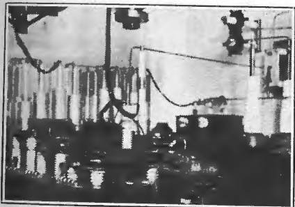
High Tension Room VIS. In the foreground are six banks of sixteen "quenched" gaps in each. In the background the Leyden Jar Condensers (12,000 cms each), with provision for using a number of series—parallel groups, according to power used. To the right the 35 K.W. transformer, and behind it the 5 K.W. transformer, with switch (controlled from operating room), for changing from low-power to buzzer; a glimpse of the latter is seen between Leyden Jars and small transformer. The bottom ends of coupling and variometer helices are seen at top of photograph.
