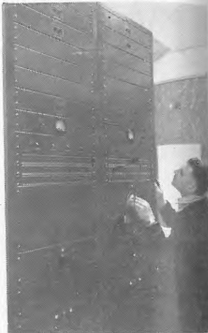
Manager of 2HD, Jim Story, shown at the controls of the amplifier racks.
