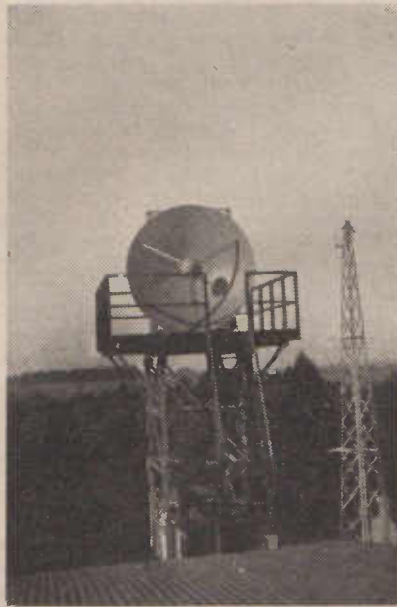
Micro-wave Parabolic antenna system as used for television relay links.
