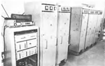
Transmitters and Power Supplies at Dural.
