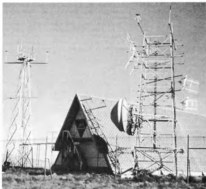
Transmitter Relay at Mount Ginini.
