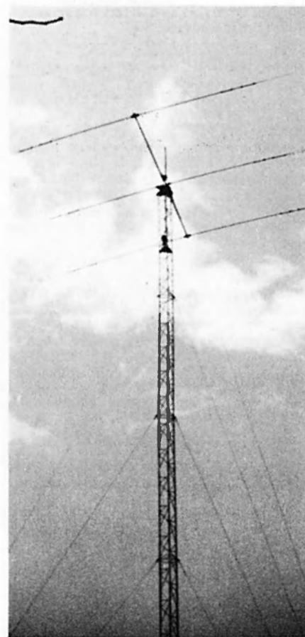
TH6 antenna at 25 metres.
