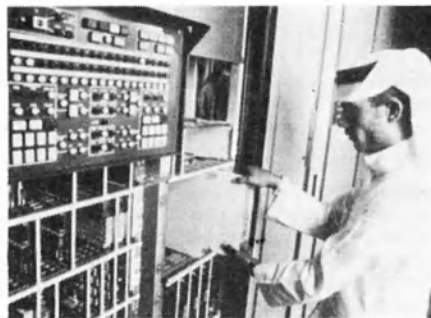
Data transmission equipment in Saudi Arabia. (Photo: Philips)
