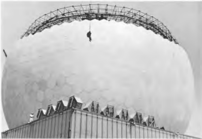
RADOME at RCA-Moorestown, to be used for testing BMEWS equipment, is 140 feet in diameter, atop a 3-story building.
