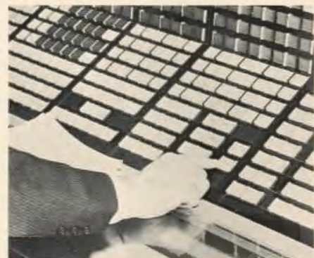
Operator monitors and controls the system's operations from the control panel.
