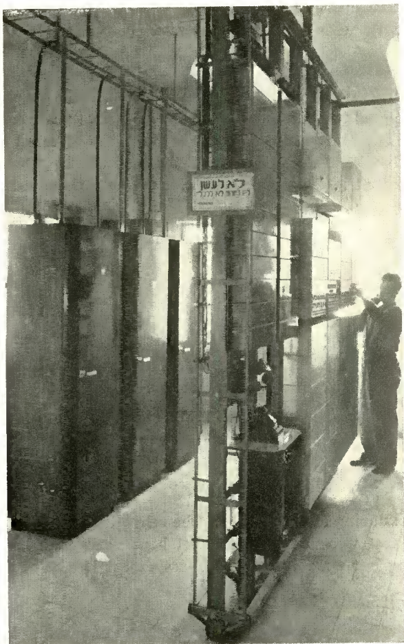
Fig. 2—Tel Aviv terminal radio and carrier equipment.
