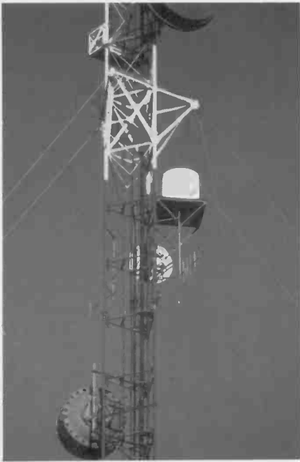
Fig. 4. Tower mounted Superquad on Long Island. A radome enclosure protects the antenna from the weather.
