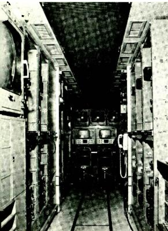
Fig. 4—Photo of rack equipments.
