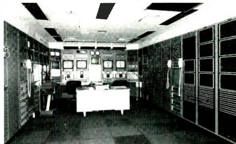
Fig. 3 — These photos compare the old master control patching bays for video (above left) and audio (above right) with the new audio and video transmission center (below).
