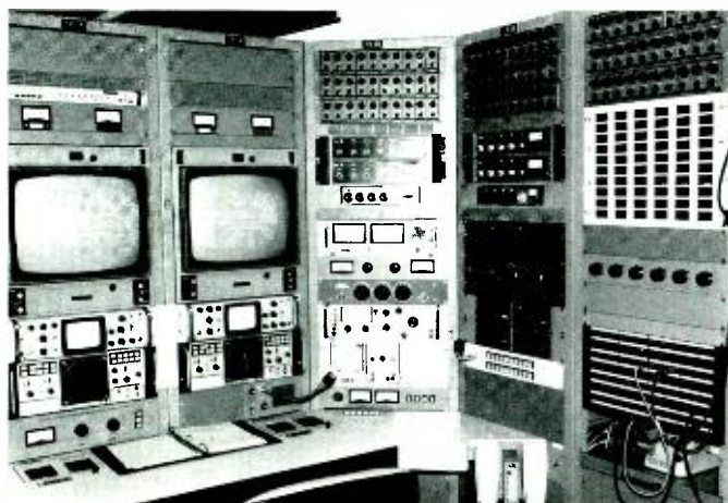
Fig. 1 — Special audio monitoring equipment (right) is conveniently located within the transmission center. The line-input monitoring selector panel may be noted at the bottom of the canted rack. The panels at the top of the three right-hand racks are input-line-level setters.
