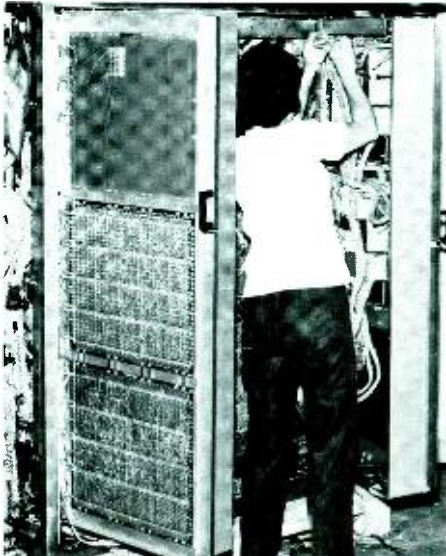
The profusion of wiring harnesses in a central processing unit (CPU) make it a "nightmare" assembly task.
