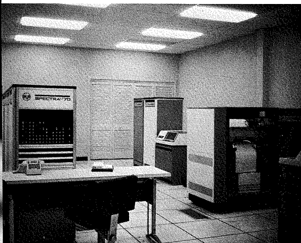
Efficient method of air distribution—conditioned air is supplied through floor grills, warm air is returned via ceiling grills (near the light fixtures).
