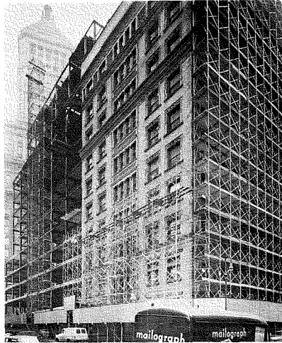
Fig. 2—66 Broad Street, Central Telegraph Office, scaffolding installed for demolition and erection of new facade.
