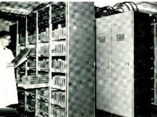
Fig. 5—Universal life-test rack for any type of component. Power-distribution panel at top allows modular expansion to any number of racks needed.
