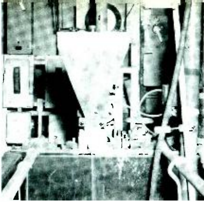
Fig. 4—The dry-feeder hopper stores and feeds filter aid, boric acid and carbon. A small stream of chemicals can be seen dropping into an electrolytic purification tank, part of a large, automatic plating machine.
