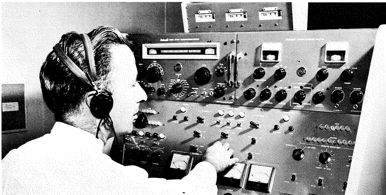
Fig. 2—In this view Niles Barlow, RCA Radiomarine Engineer, is shown at another control console arrangement that handles shipboard communication between SSB transmitter, remote receivers and the shipboard telephone switchboard.
