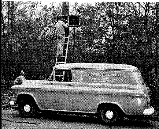
Fig. 4—Repeater amplifier under installation test by Charles Collins while Frank Hensley, supervisor from RCA Service Company observes.
