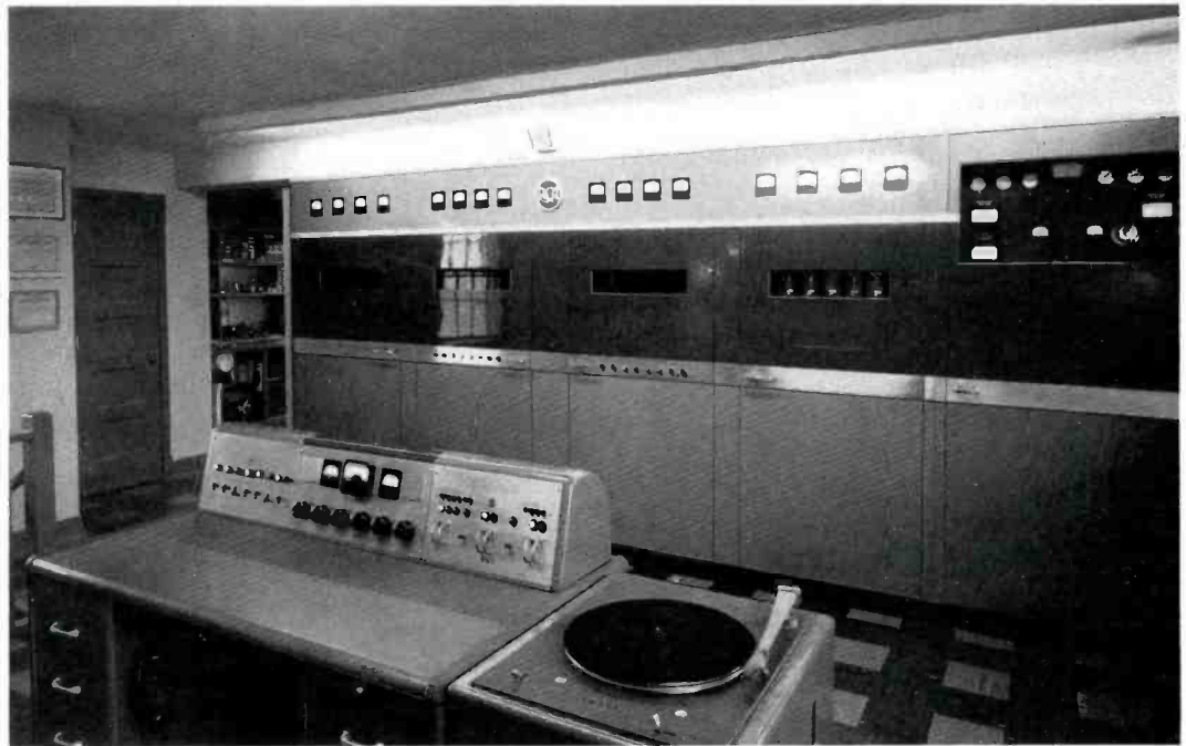
FIG. 6. Front view of the KOTA 5-KW AM Transmitter, RCA BTA-5F, and Companion Supervisory Console.
