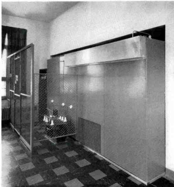
FIG. 7. Rear view of the AM Transmitter at KOTA showing an unusual space-saving enclosure for high-voltage components which leaves the major portion of the room free for other uses.
