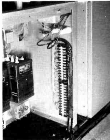
FIG. 11. View showing inter-connecting cables and terminal board "tie" connections.
