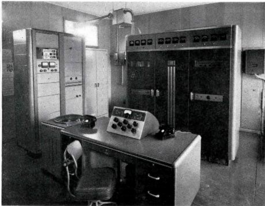
FIG. 11. View of the KOZY 3-KW FM Transmitter, RCA BTF-3B and Associated Console and Monitoring Racks.
