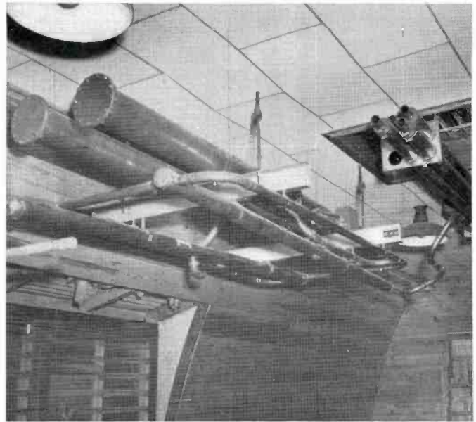
FIG. 12. The Notch Diplexer and Side-Band Filter in the TV transmission line are ceiling mounted units of the new simplified design.
