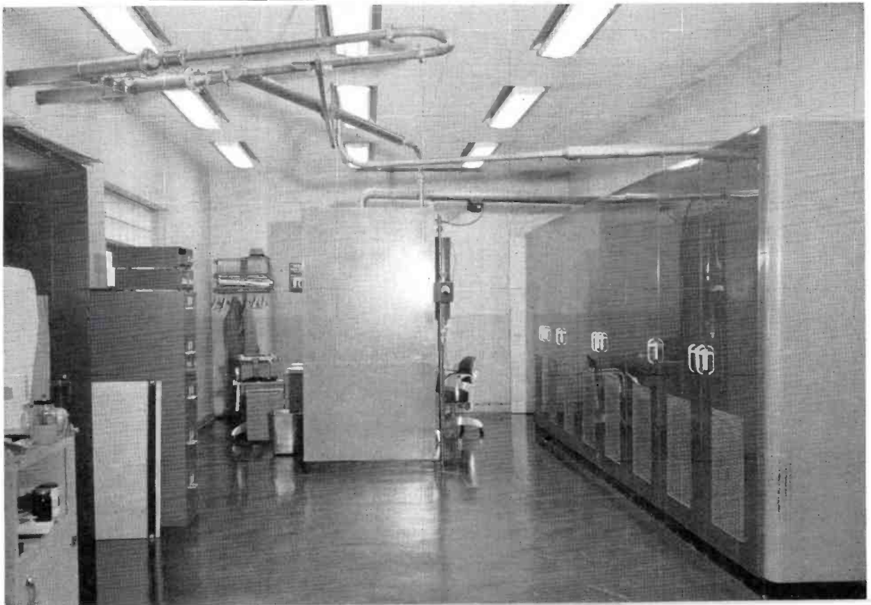
FIG. 3. Above floor plan shows arrangement of TV transmitter and studio facilities. Plans call for expansion of TV building to include new TV studios and WDAF AM studios. Below is a rear view of the TT-5A, with vestigial sideband filter (center) and diplexer mounted overhead.
