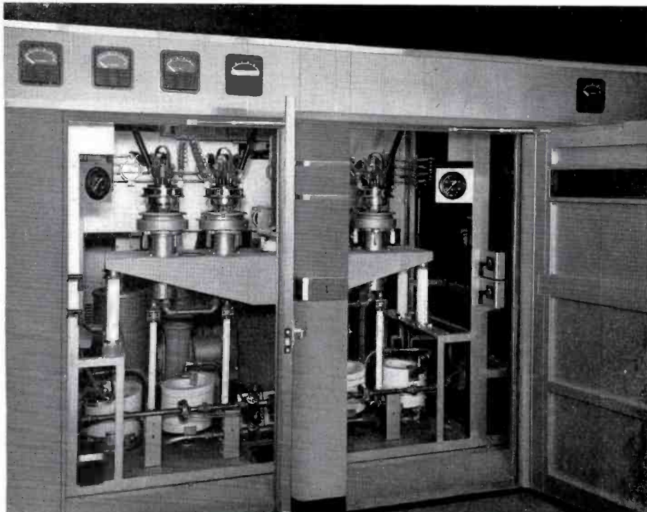
FIG. 10 (below). In this view doors to the 150 KW power amplifier are opened to illustrate the assembly of the four 9C21 power tubes on a single base plate.
