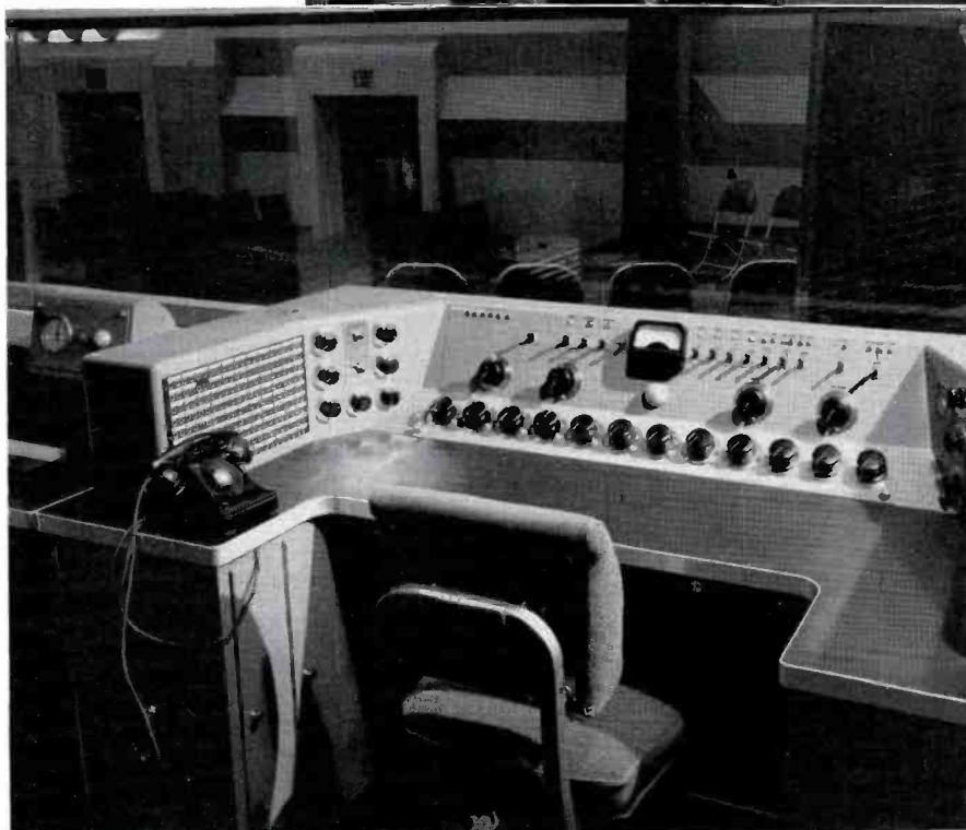
FIG. 6 (below). This custom-built studio console provides complete facilities and operating convenience for the control of auditorium type studio "A". Identical equipment is also employed in large studio "B".
