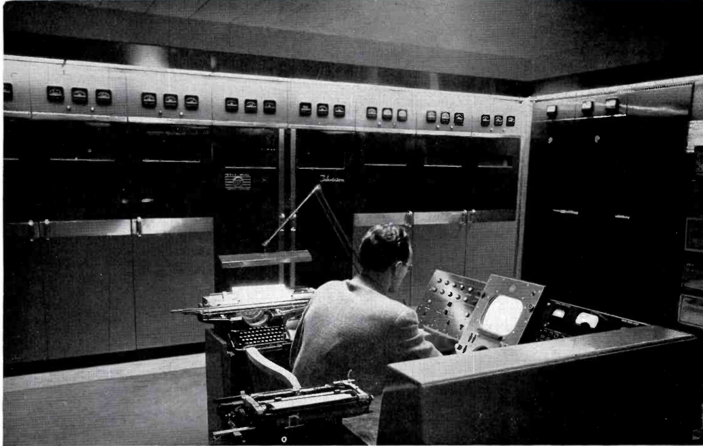
FIG. 27. WCAU-TV's Transmitter (RCA Type TT-5A) is shown here (left background). Monitoring racks are at the right, control console in the foreground. This photograph is taken from a position just in front of the FM transmitter (see floor plan. Fig. 25).
