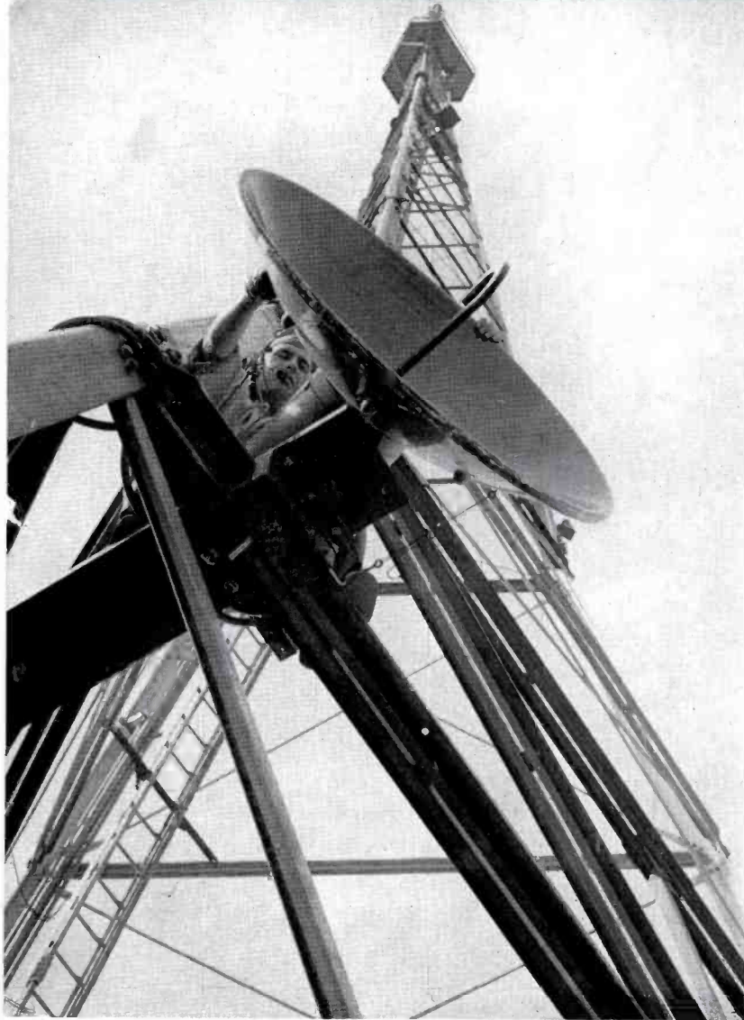
FIG. 31. WCAU-TV's exceptionally high tower is an ideal location for the RCA TTR-1A relay receiver used to pick up video signals from the mobile unit. The parabola shown above is mounted so that it can be oriented through a wide angle. Other positions provide for pickup from all directions.
