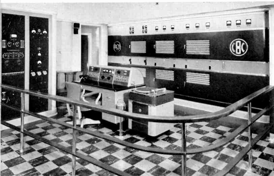
The RCA 5-DX and associated equipment installed at CBM.
