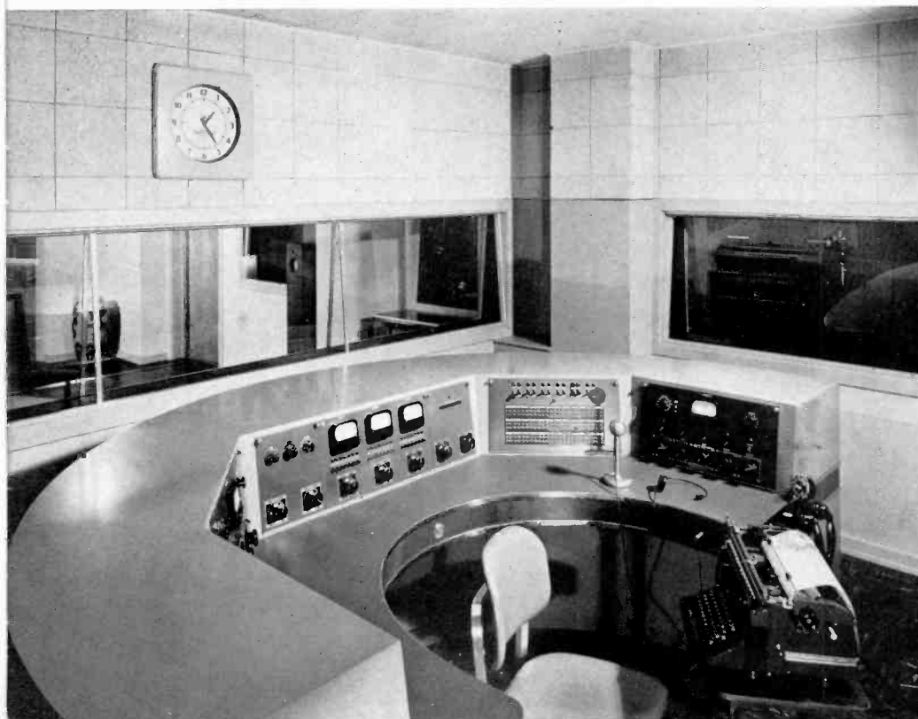
Master Control Desk at WIRE.
