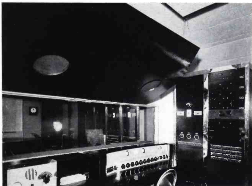
Figure 4. Studio Control Room Equipment.
