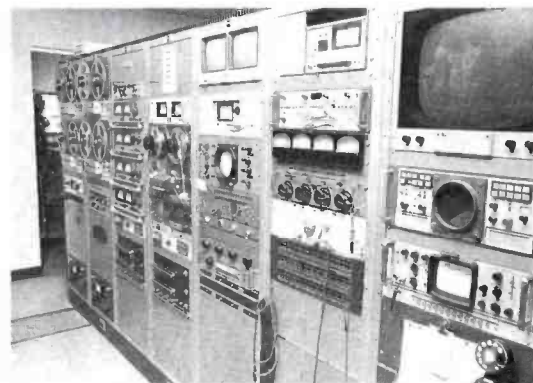
Equipment racks behind operator position.
