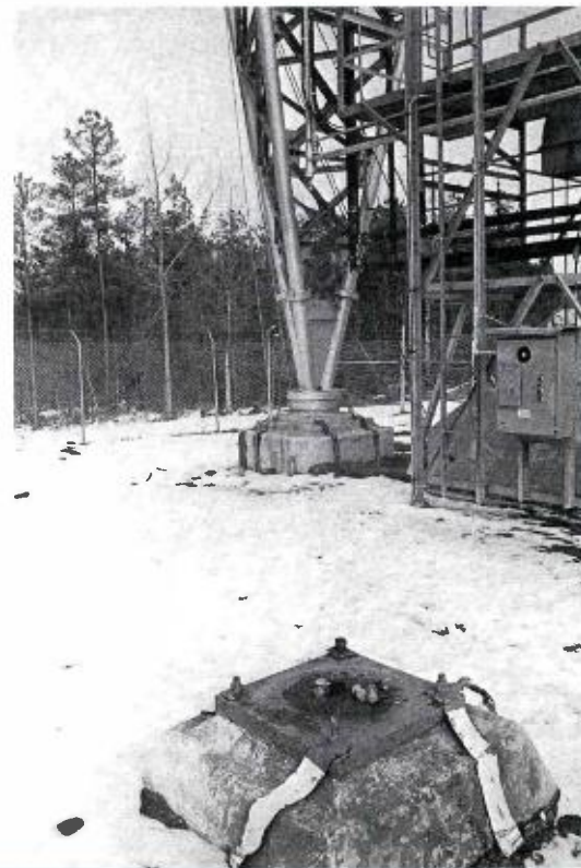
Base of dismantled old tower in foreground. New tower was erected within 30 feet of the existing tower.
