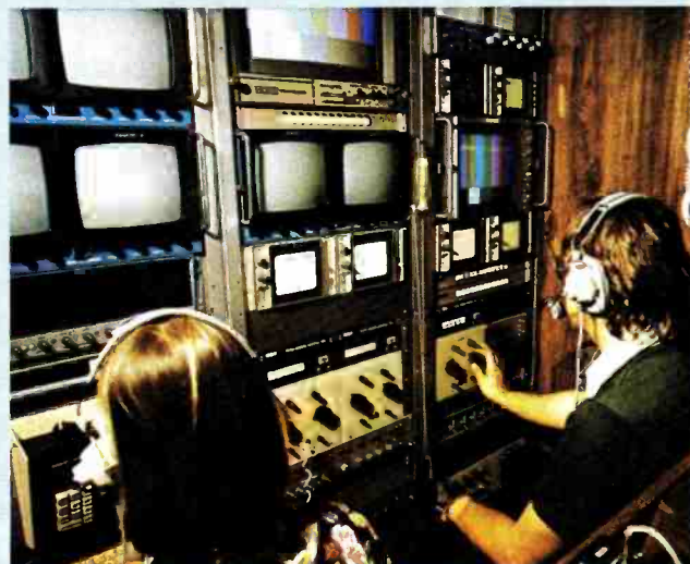
Graphics and-video-control operating positions in front of monitor, test and distribution racks.
