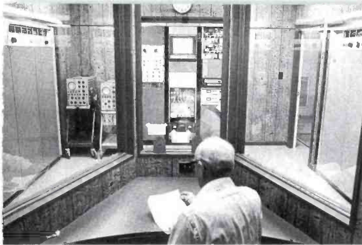
Transmitter engineer in noise-isolated "booth" has full view of TV and FM transmitters and monitoring equipment.
