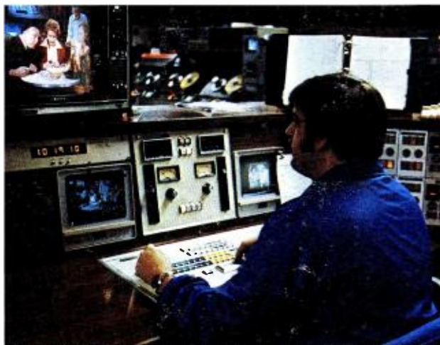
Master Control On-Air switching console, with tape machines in background.
