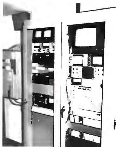
Satellite Earth Station operated by TV-11 is mounted on an adjoining parking garage roof. System uses an 11-meter Steerable Receiving Antenna and provides access to TV newscasts originated by ITNA-affiliated stations. Rack equipment for the Earth Station is conveniently located in the Technical Area near Master Control.
