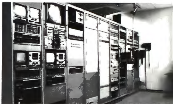
Monitor, control and terminal equipment racks. Camera CCU's are to be relocated in a console.
