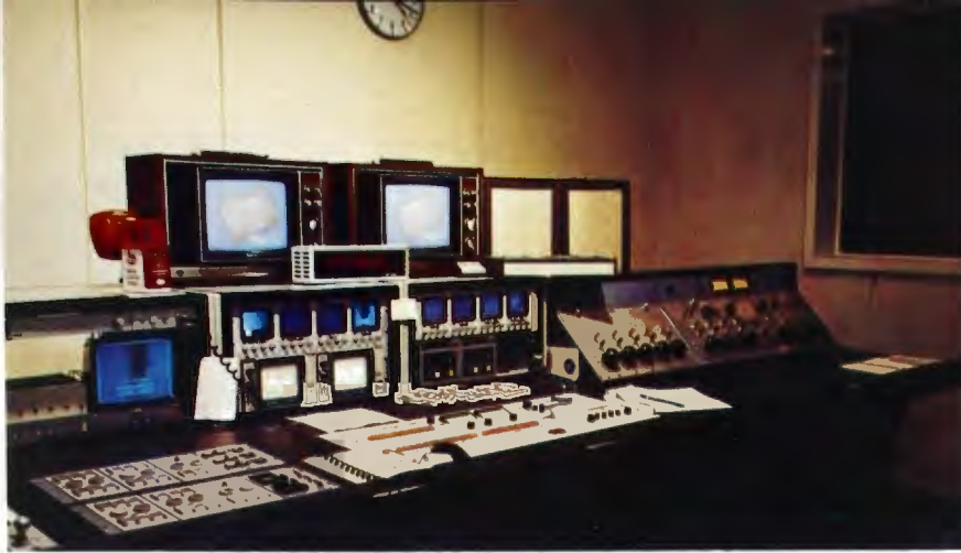
Master Control Room.
