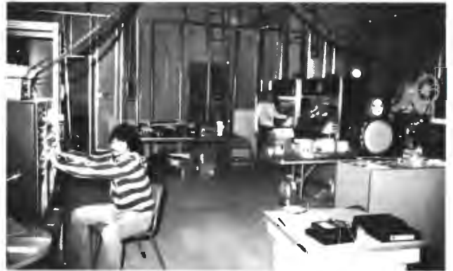
Addition of a TK-28 telecine island and two TR-22 VTR's moved TV-4 into full local and network programming and commercials.
