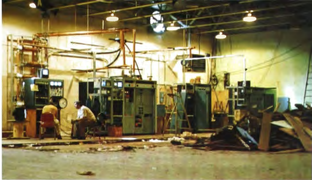
The major effort was in getting the TV station on-air for the 1977 baseball World Series. Even amid the debris of converting the sports arena into a broadcasting station, the TV transmitting system aired the first game. At left is the makeshift "master control" with the oversize clock.
