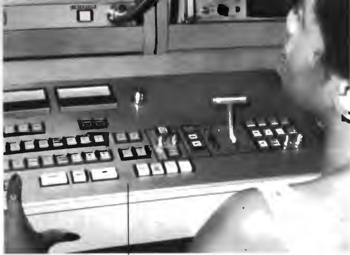
TV-11 Master Control console puts the operator in command. Unique, station-designed push button arrangement at bottom of MC switcher simplifies operations while minimizing errors.
