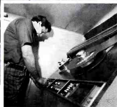
TR-600 mounted inside TV-20 van provides top quality recordings. One engineer handles the taping operating and shades camera on remotes.
