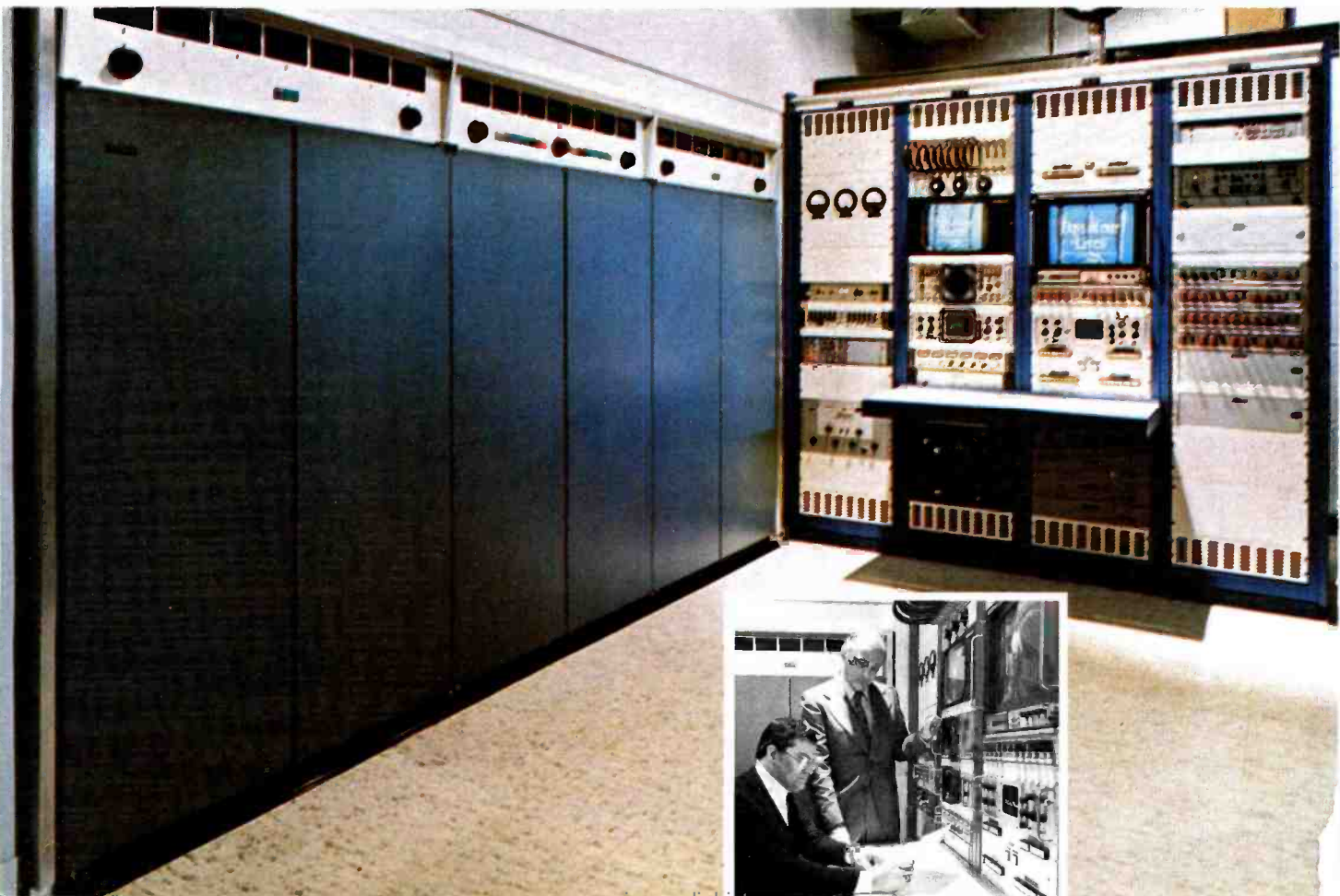
Front line cabinets of TT-50FL, 50 kW transmitter at WKYC-TV are built-in to form a wall of the control area. Extending at right angles to the transmitter are the audio and video monitoring racks.
