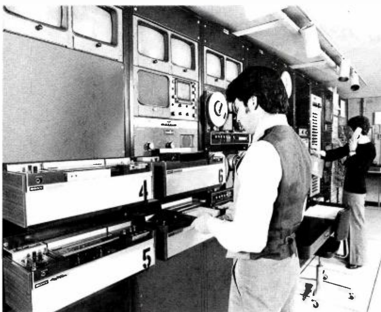
"House" TV distribution system permits sending up to eight video programs simultaneously to 150 locations throughout Merrill Lynch headquarters.
