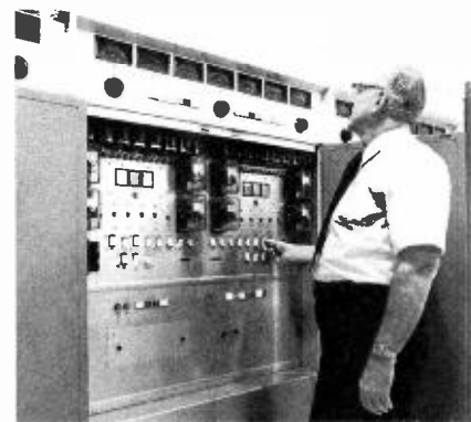
At the combined control cabinet of the TT-50FL is Kirk (Sandy) Sanderson, Transmitter Technical Director for WKYC-TV, who handled many of the system installation and check-out operations.
